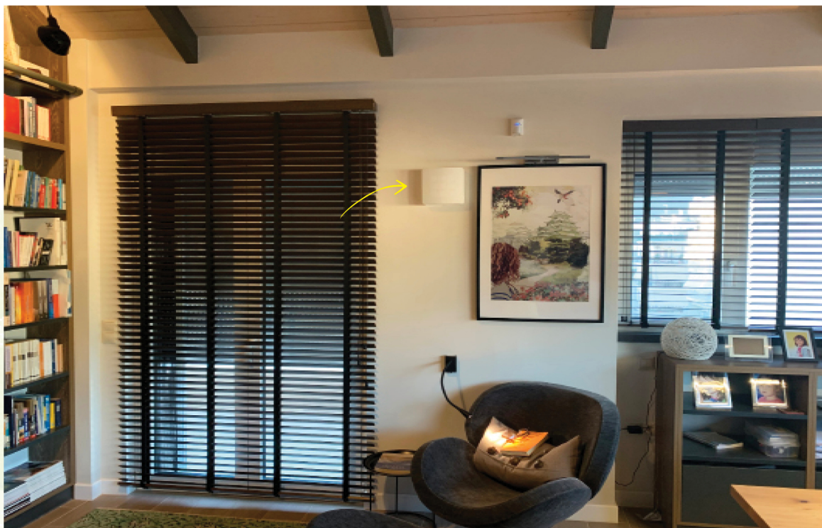
Heat recover ventilation at a house's library space
